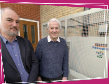
Guy Ransom, of Finn Geotherm with Cllr Gerald Kelly, Cabinet Member for Governance, Regulatory and Environment, looking at heat pumps.
